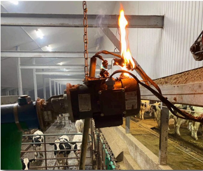
Damage to a cable caused by the vibration of a motor.
