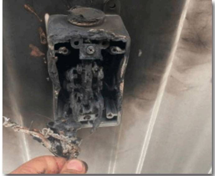
Major fault in an electrical outlet, caused by moisture and corrosion.
